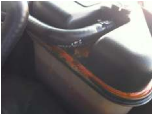
Figure 1 Top overflow line attached to plastic nipple on top of tank
