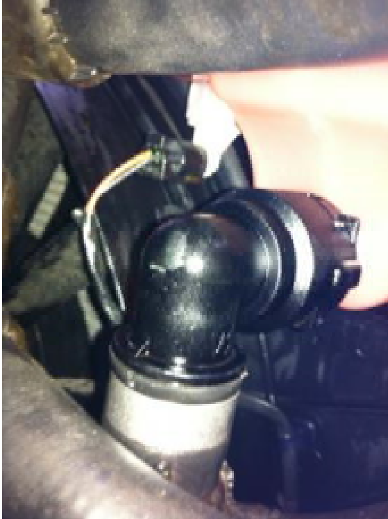
Figure 2 Level Sensor (Left) and Primary Overflow Line (Right) attached to bottom of tank
