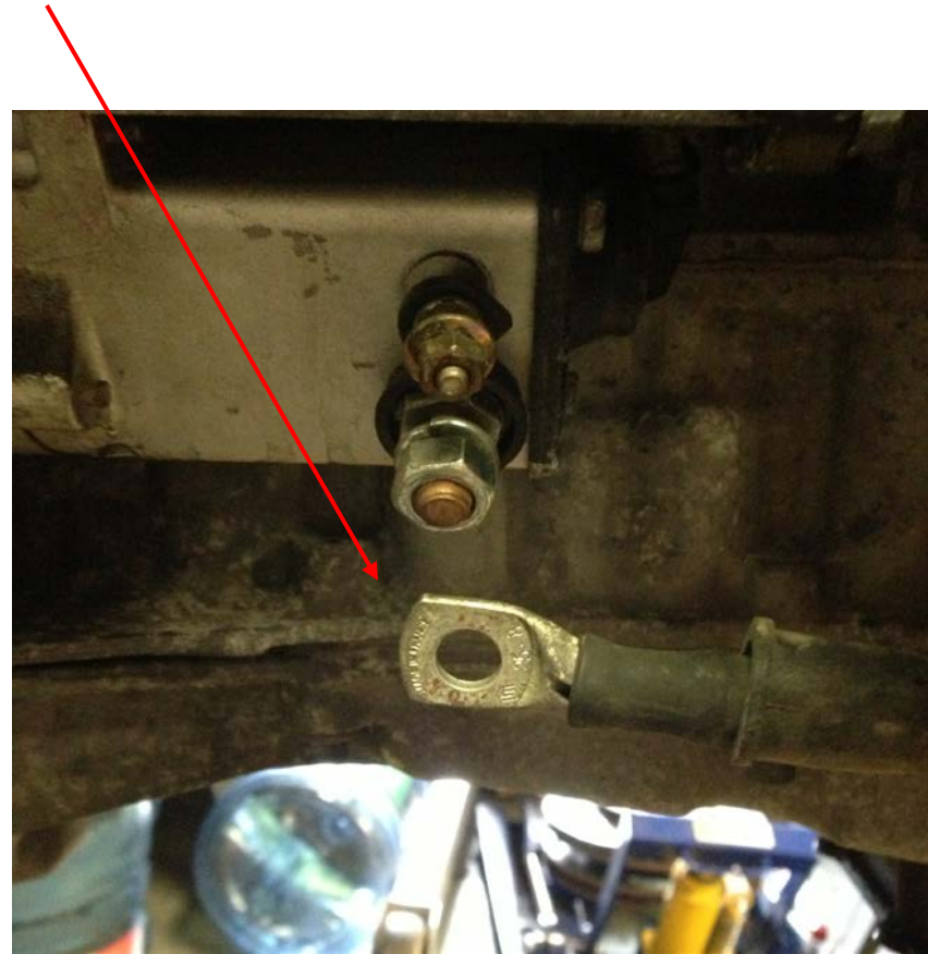
Starter connection (other end of the same cable)
