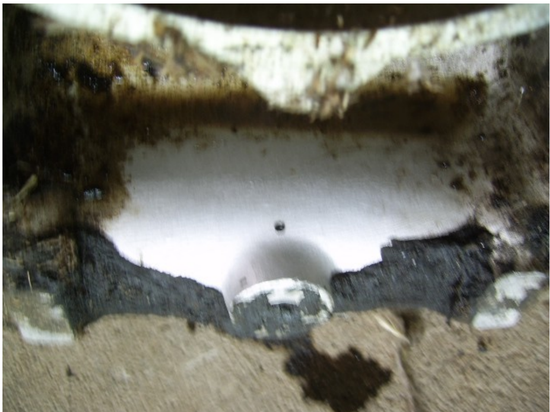
Figure 2 Close up of said hole
